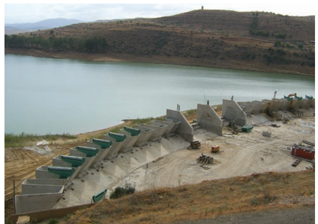
Close view of Ghrib Fusegates
