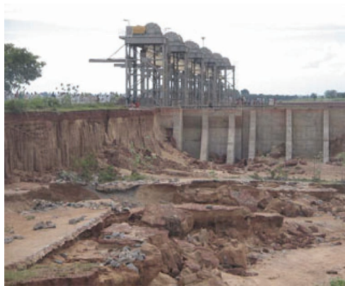
The collapsed embankment and spillway
