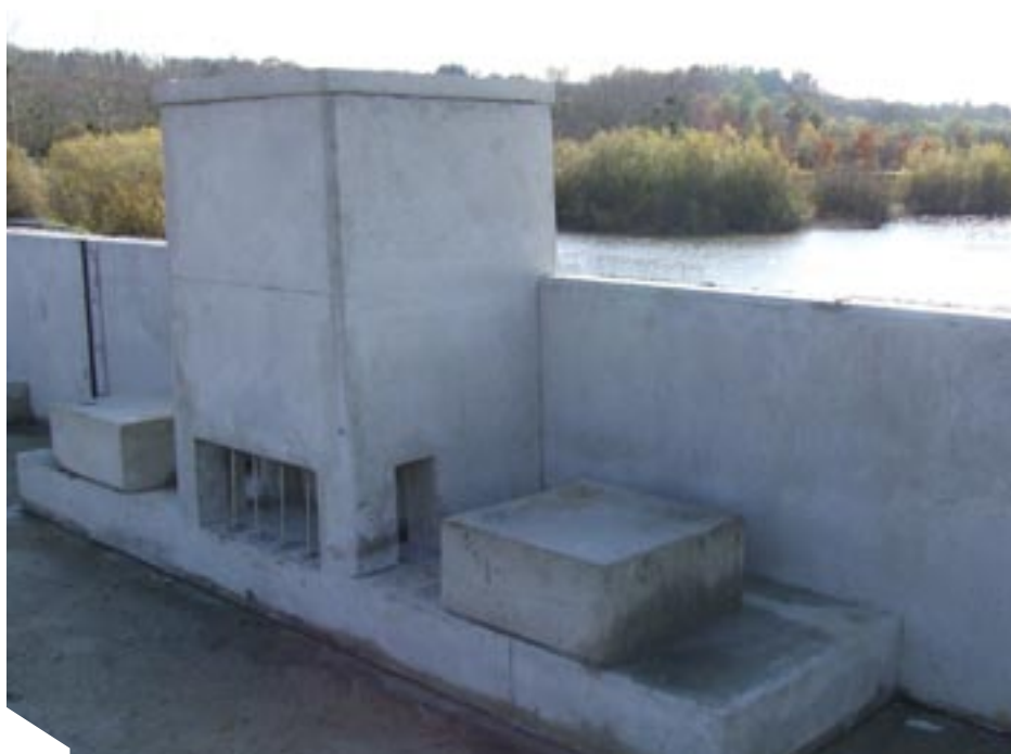
Close-up view on the Allan fusegates and their special well structure preventing vandalism.
