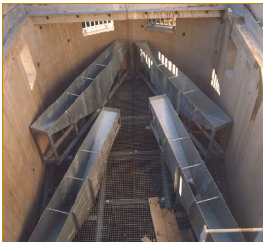
INSIDE VIEW OF THE PROTECTIVE ENCLOSURE FUNNELS, LINKED TO THE FUSEGATES BY EMBEDDED PIPES
