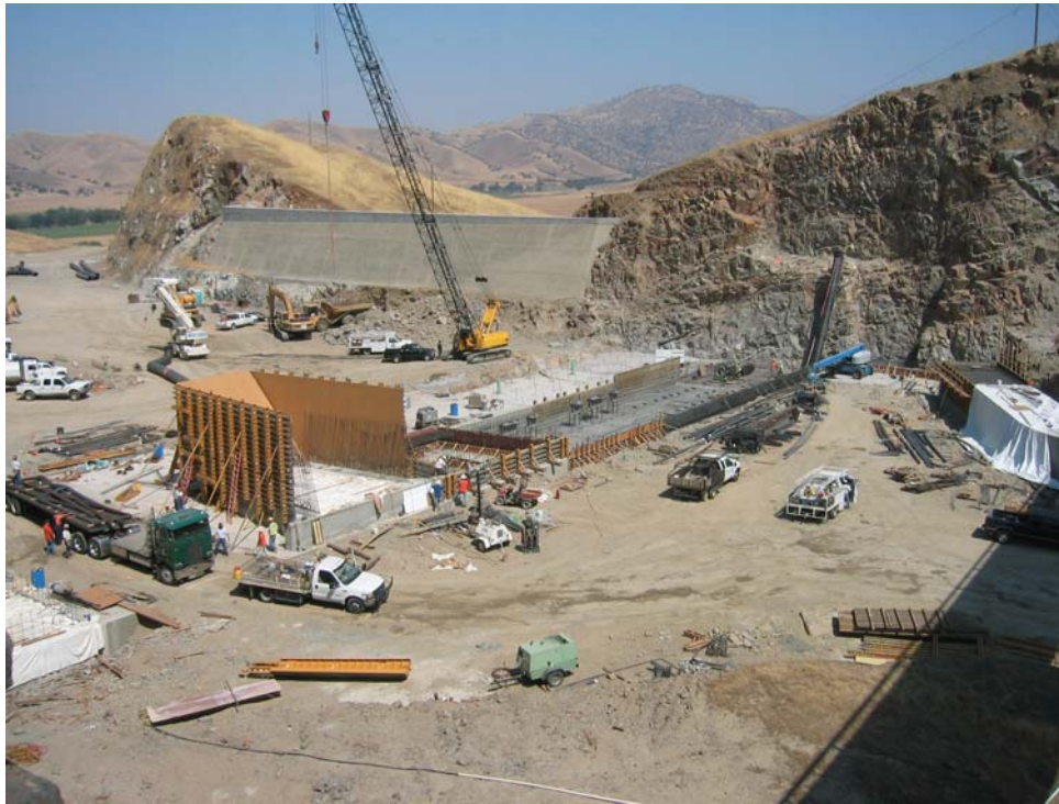
Figure 8. Installation of Fusegate formwork for lateral walls and the pipes in the foundation
