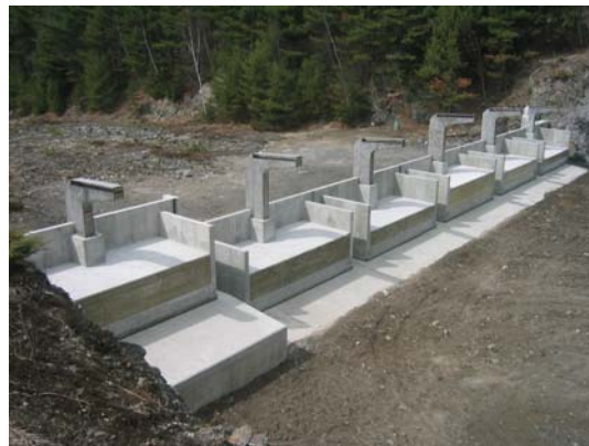
Fig. 9 Downstream view of Fusegates
